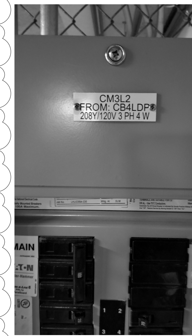
EXISTING PANEL IN SKYVIEW IT ROOM
