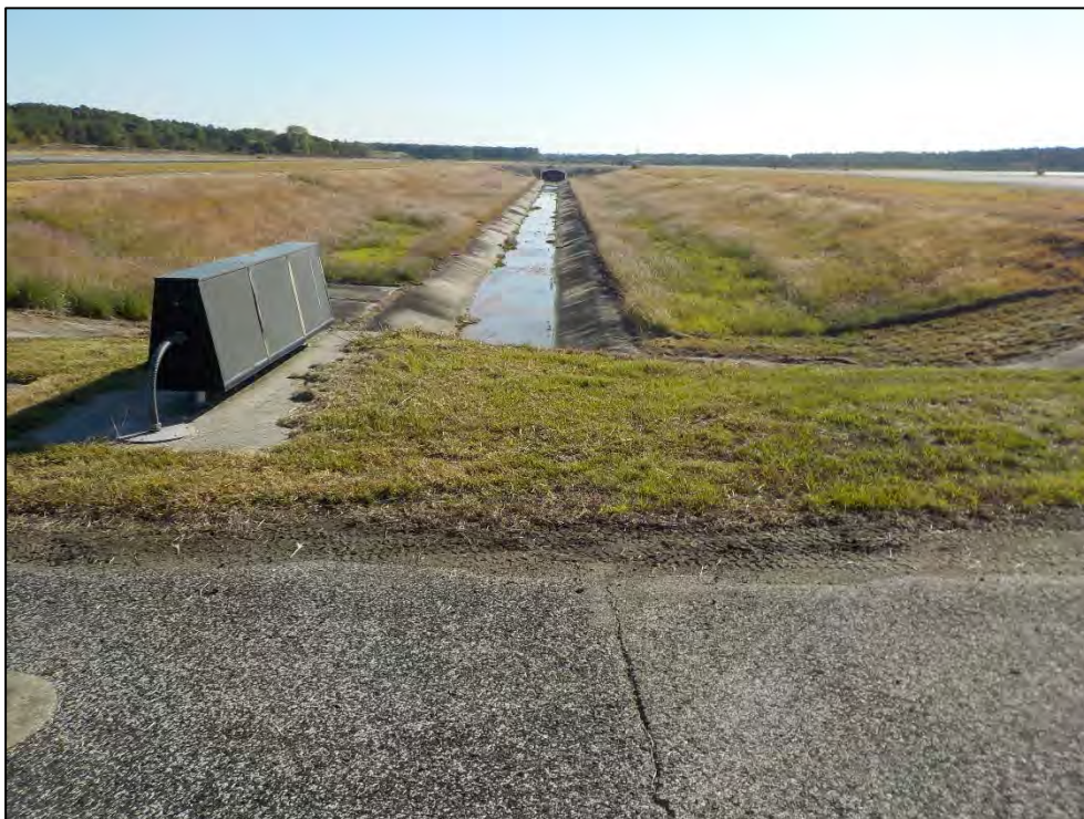
Photo 12. Overview of the drainage ditch between the Taxiway SA and SB near the east end, facing east.
