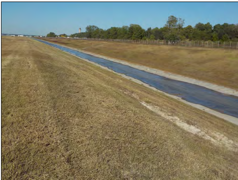
Photo 10. Overview of the northern drainage ditch (north of Taxiway SA) at the east end, facing west.
