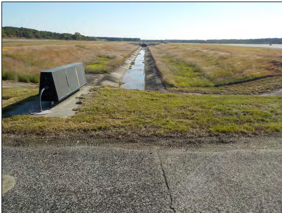
Photo 14. View of the drainage ditch between Taxiway SA and SB near the east end, facing east.
