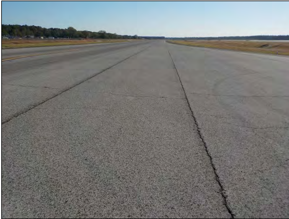
Photo 9. View of Taxiway SA near the center of the project area, facing east.
