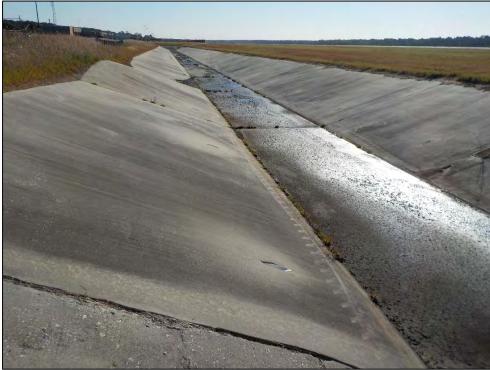
Photo 9. Overview of the northern drainage ditch (north of Taxiway SA) at the west end, facing east.
