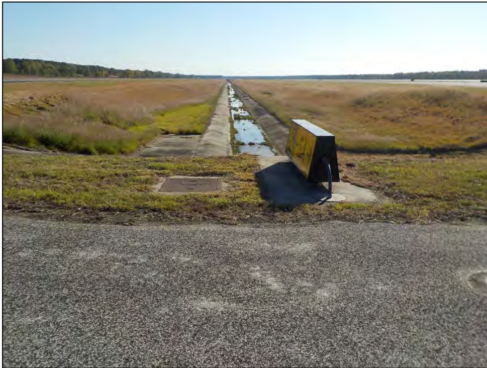
Photo 11. Overview of the drainage ditch between the Taxiway SA and SB at the west end, facing east.
