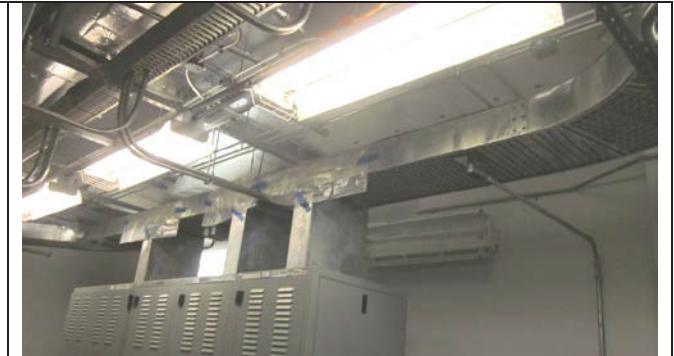
General view of APM Equipment Room (A407). Note poly over the cable trays
