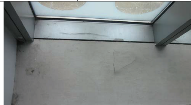
Example of observed water staining on window sill on the APM Level
