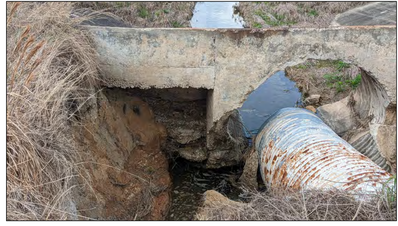
② EROSION DAMAGE
