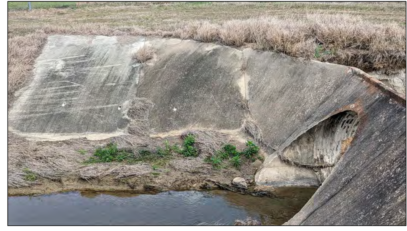
① CONCRETE GROUT FAILURE
