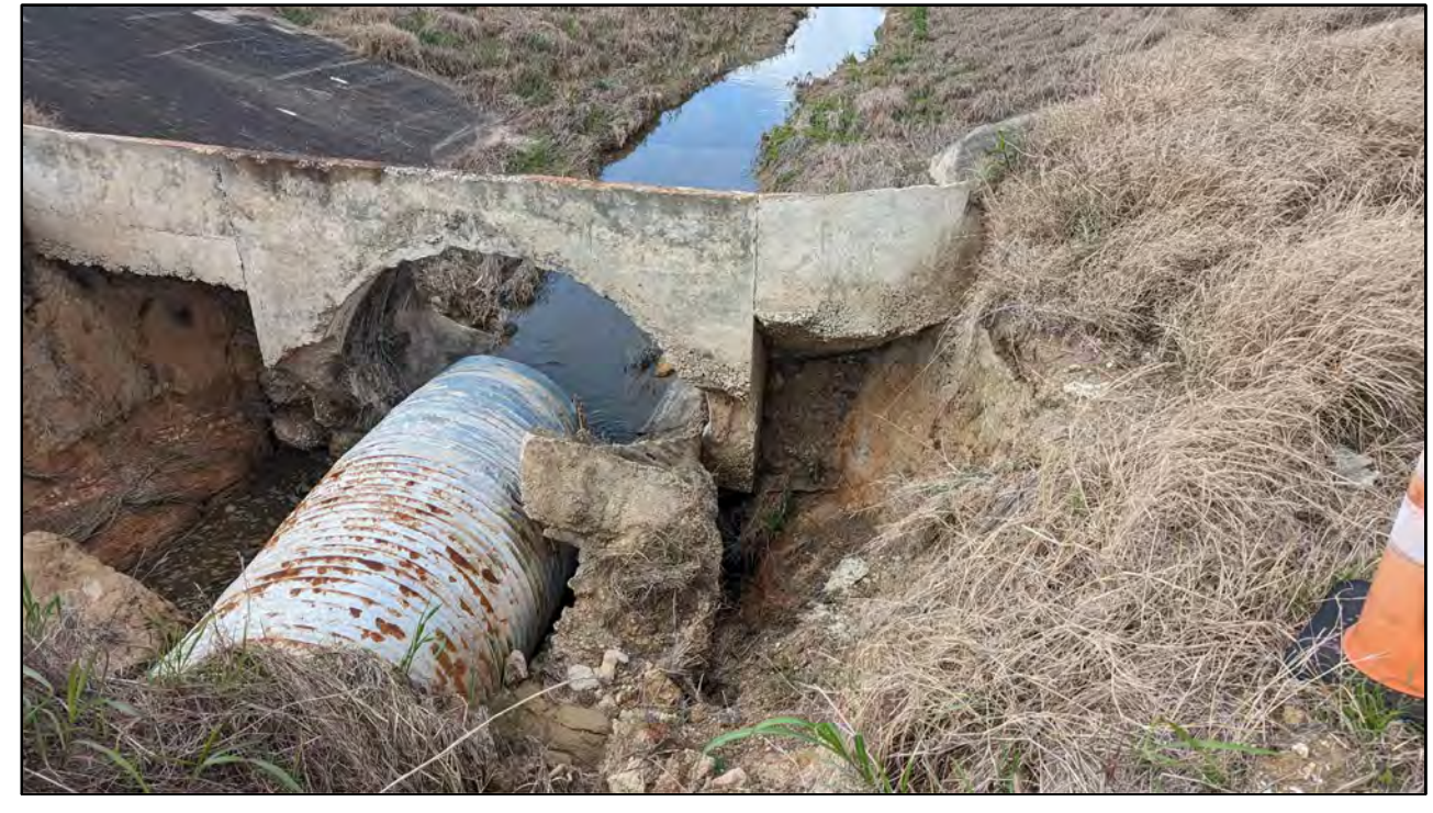
③ EROSION DAMAGE
