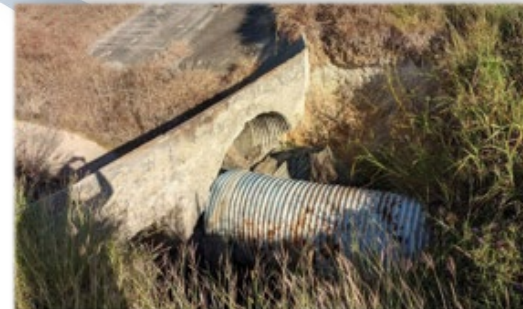
Figure 4 – North Culvert Headwall Erosion
