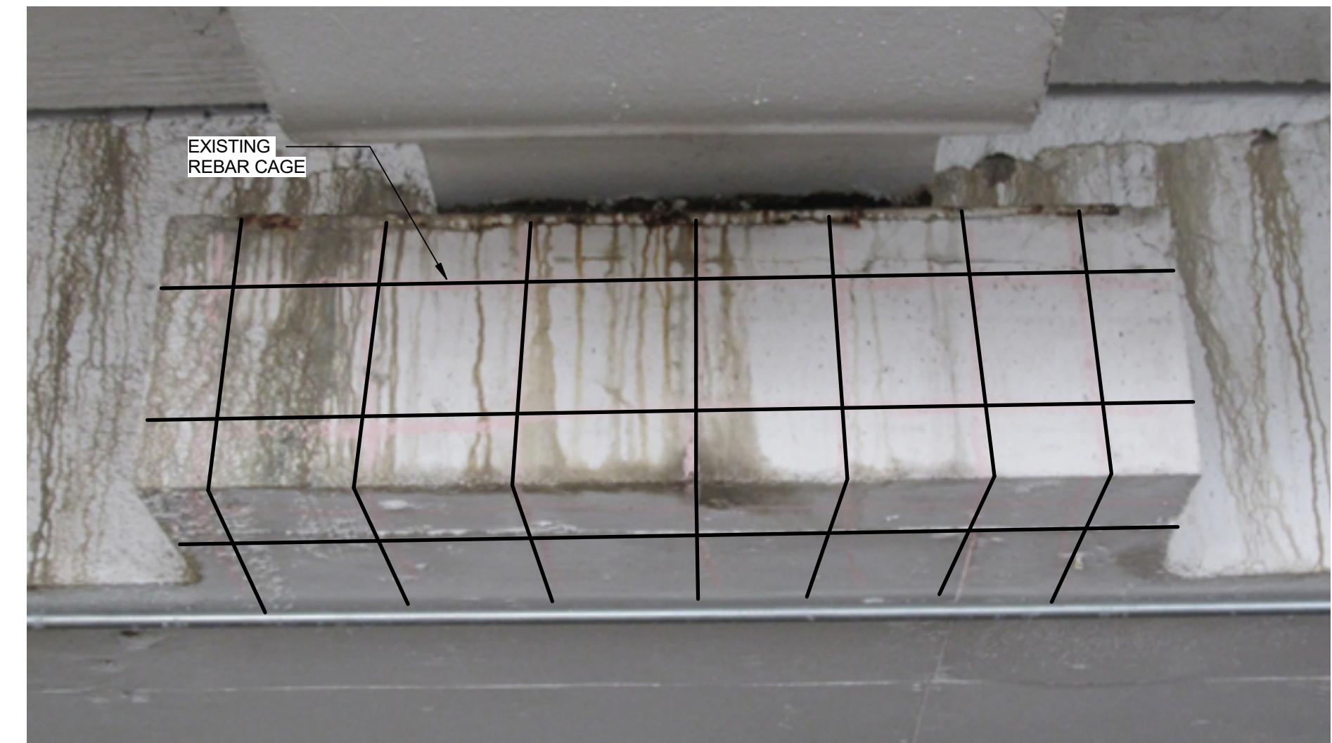
11 EXISTING CORBEL - REBAR IDENTIFIED DURING GPR TESTING (Approximate Locations) NTS
