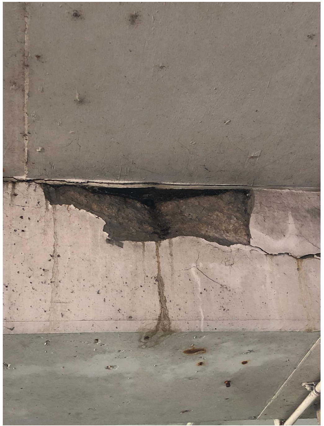
2 CONCRETE SPALLING AT RAMP BEAM SCALE: 3" = 1'-0"
