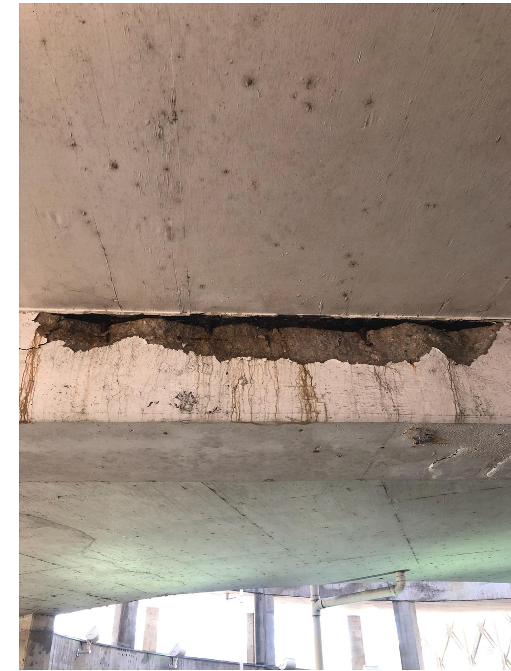
1 CONCRETE SPALLING AT RAMP BEAM SCALE: 3" = 1'-0"
