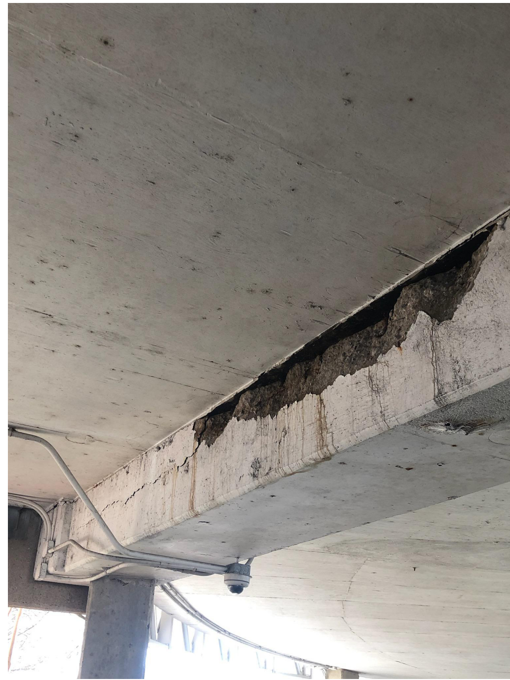
4 CONCRETE SPALLING AT RAMP BEAM SCALE: 3" = 1'-0"
