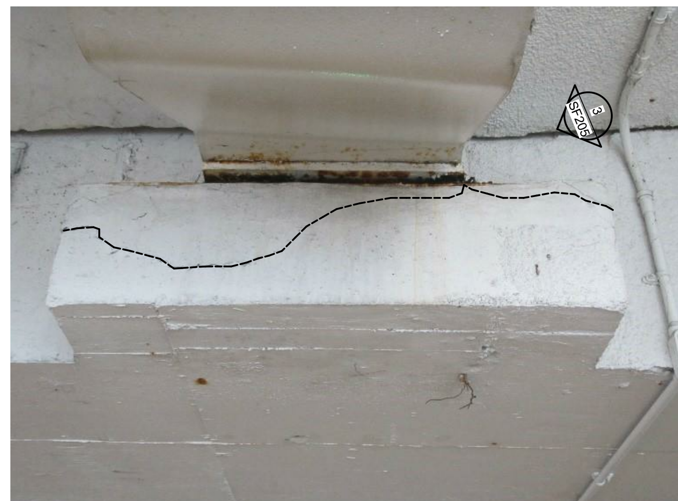
5 CRACKED & DELAMINATED CONCRETE AT CORBEL NTS
