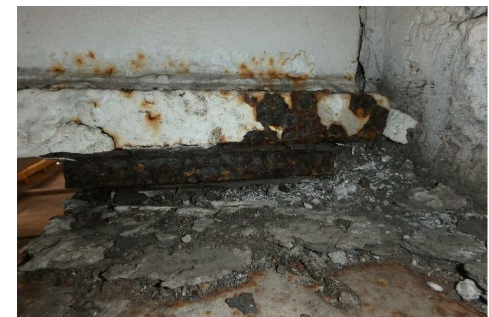
3 CORRODED STEEL PLATES IN SLIDE BEARING ASSEMBLY NTS
