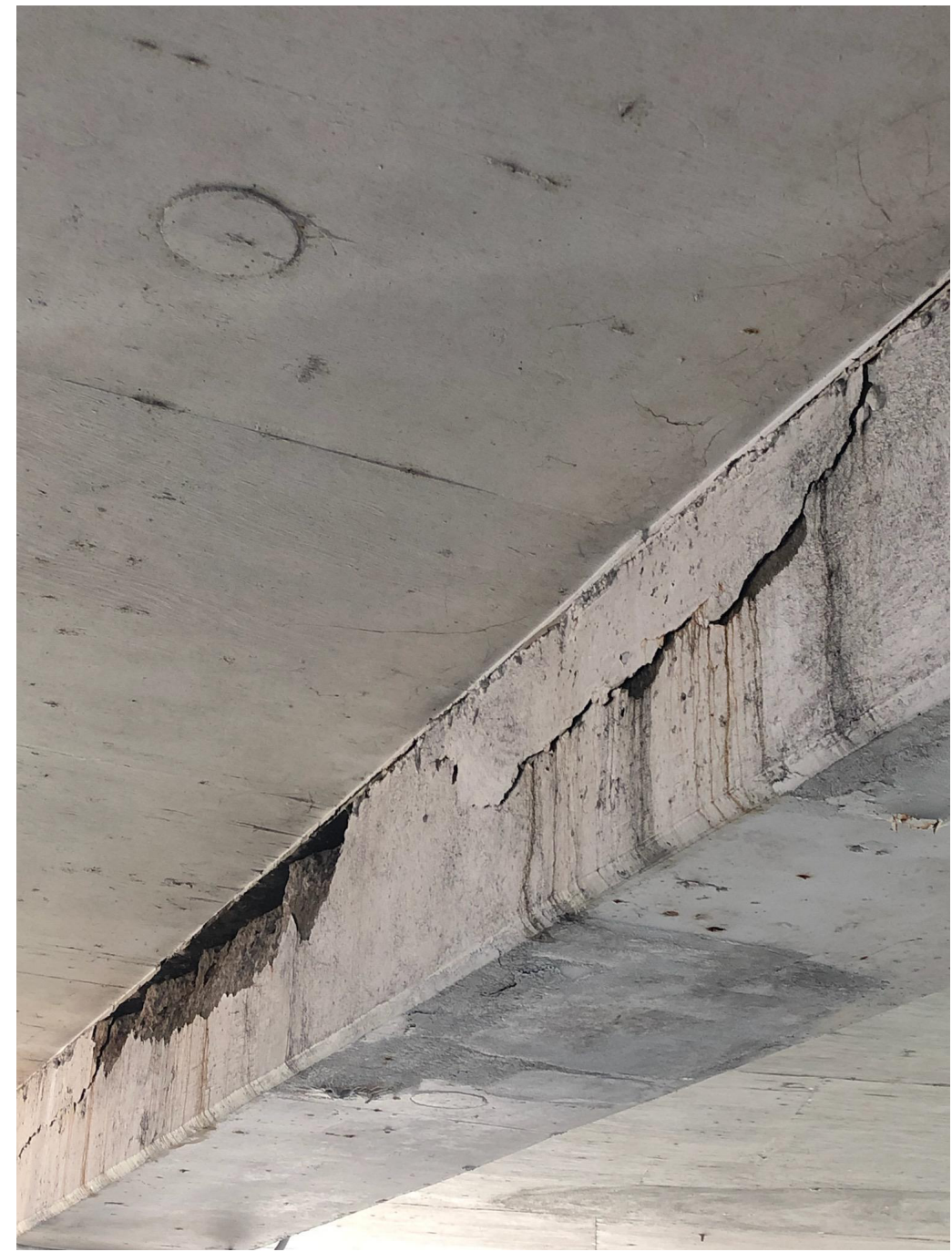
3 CONCRETE SPALLING AT RAMP BEAM SCALE: 3" = 1'-0"
