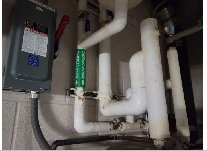
Photo 10: View of water heater room.
