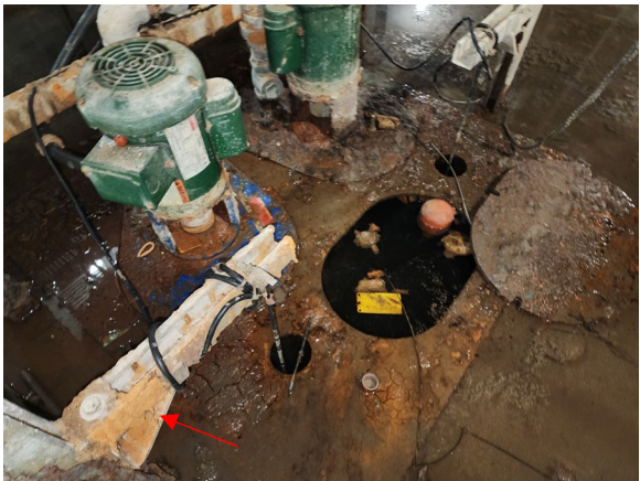
HA 13: Rust/Insulation on Truss
