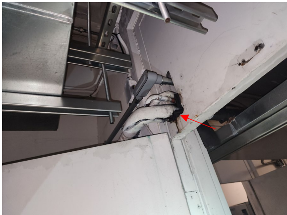
HA 8: HVAC Drain Line Insulation
