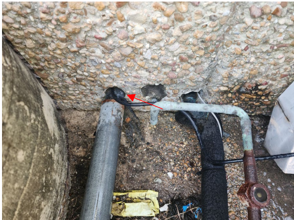
HA 10: Black Exterior Penetration Mastic (ASBESTOS DETECTED)
