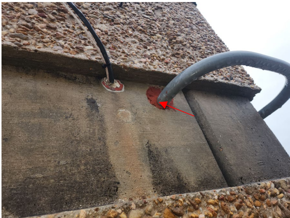
HA 9: Red Exterior Penetration Firestop
