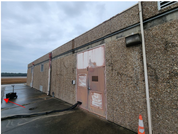
HA 7: Gray Exterior Slab Expansion Joint (ASBESTOS DETECTED)
