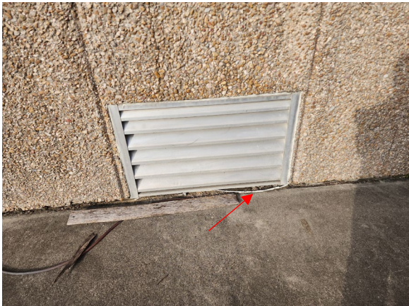
HA 11: White Exterior Vent Caulking (ASBESTOS DETECTED)
