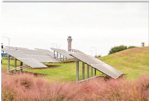
Solar panels near the IAH Central Utility Plant
