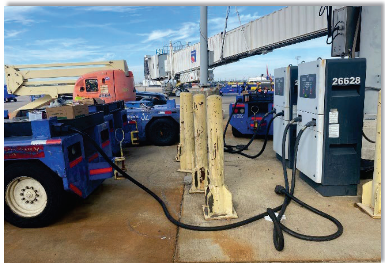
Southwest Electric GSE charging at HOU
