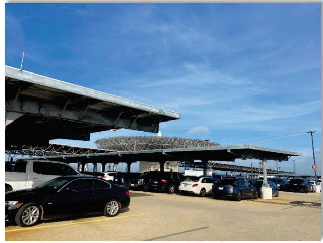
Solar array on the HOU Red parking garage
